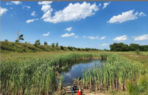
Failed Infiltration Basin, Delaware
