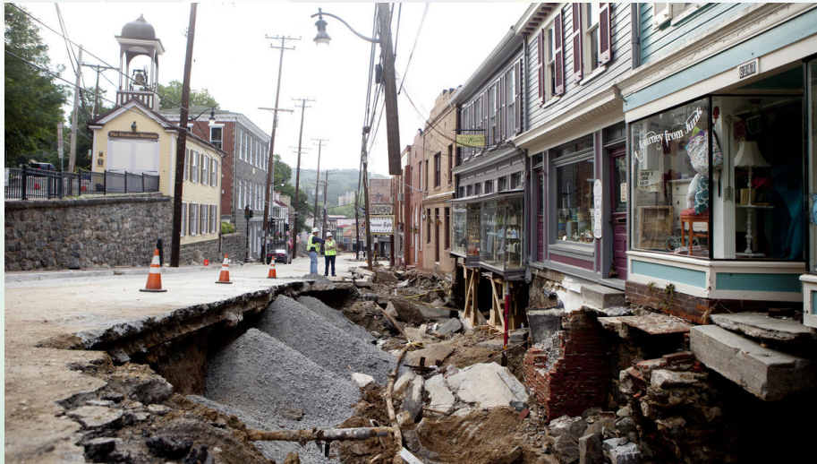
Sidewalk washed away from store fronts
