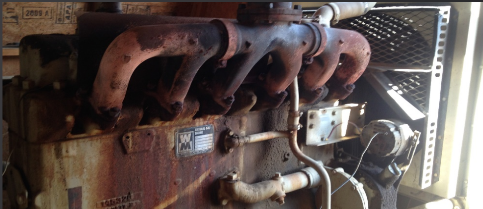
Corroded engine generator at a dairy farm
