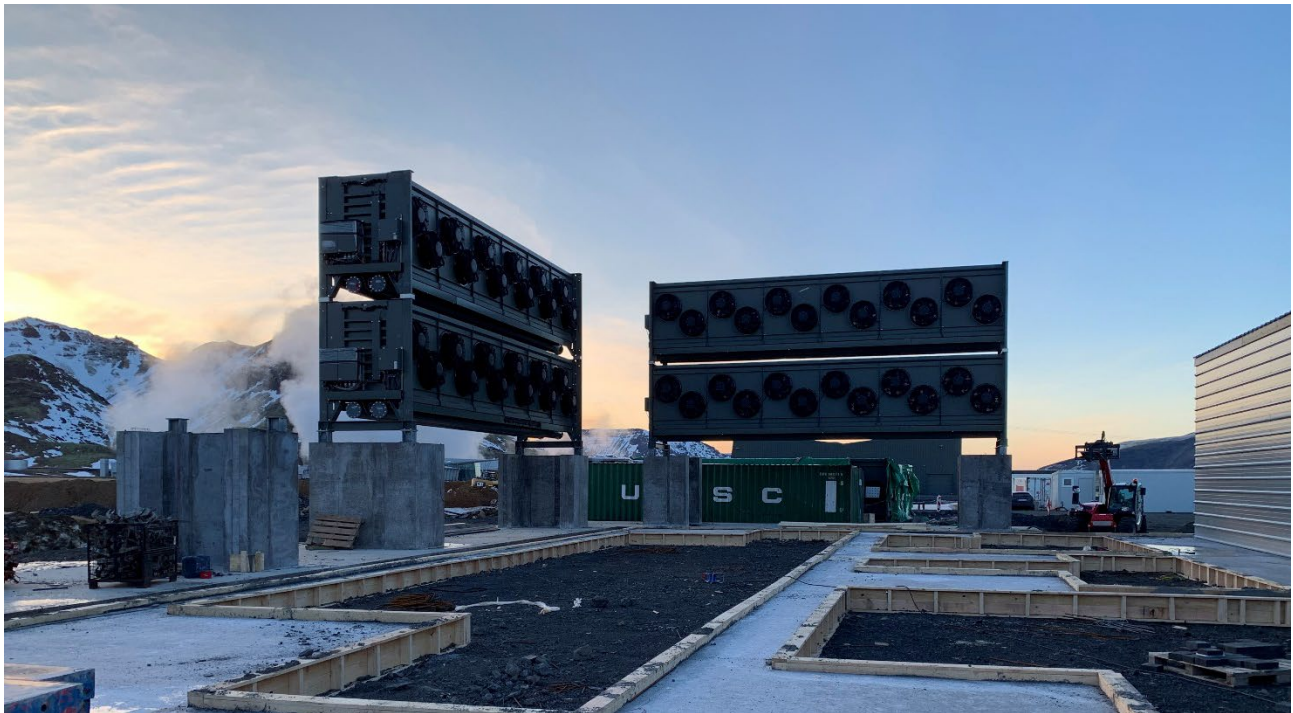
Under construction: Climeworks' new large-scale direct air capture and storage plant "Orca" (Credit: Climeworks)
